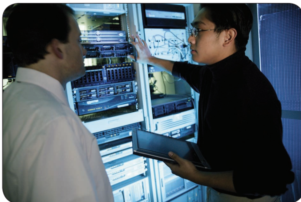
Computer technicians at work in a server room. IBM's competency centers customize teams of workers who can manage their own tasks.
